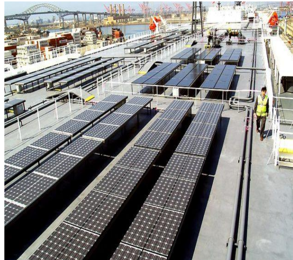
Figure 2: Installed solar panels, on Auriga Leader's deck
